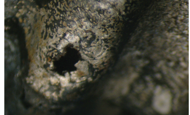
Stereomicroscope photo taken by Goodson Engineering of CSST perforation caused by lightning.
